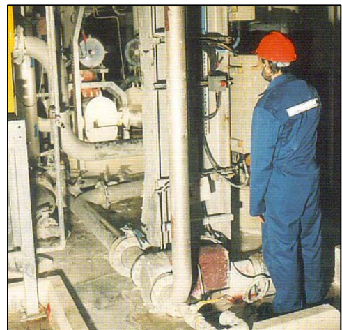
Series S pump in foreground on clay recovery Series A pump in background on paper coating
